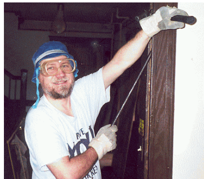
Dave Sica saves a section of chestnut trim from the New Brunswick station. Hundreds of terra cotta roof tiles were also saved for "spare parts" for InfoAge.
