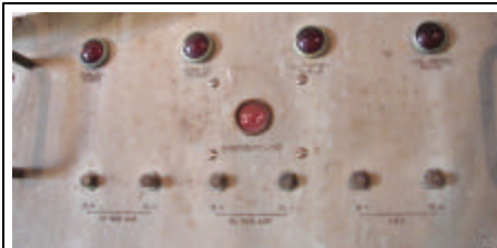
The original antenna control panel.
