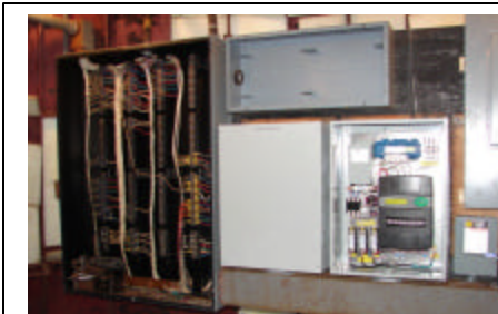
Restored control panel funded by Princeton University and worked on by NJARC member Bob Pilcher.
